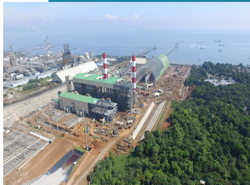
LIMAY 4X150MW POWER PLANT
